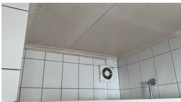
Fuktmerker i himlingen
