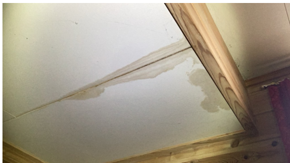
Fuktmerker i himling under bad.
