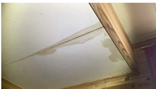
Fuktmerker i himling under bad.
