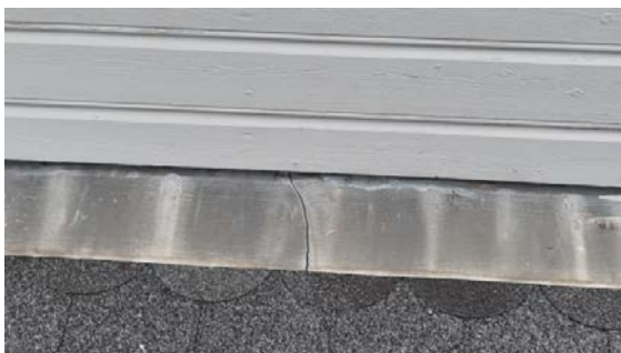
Sprekk i blyteking.
