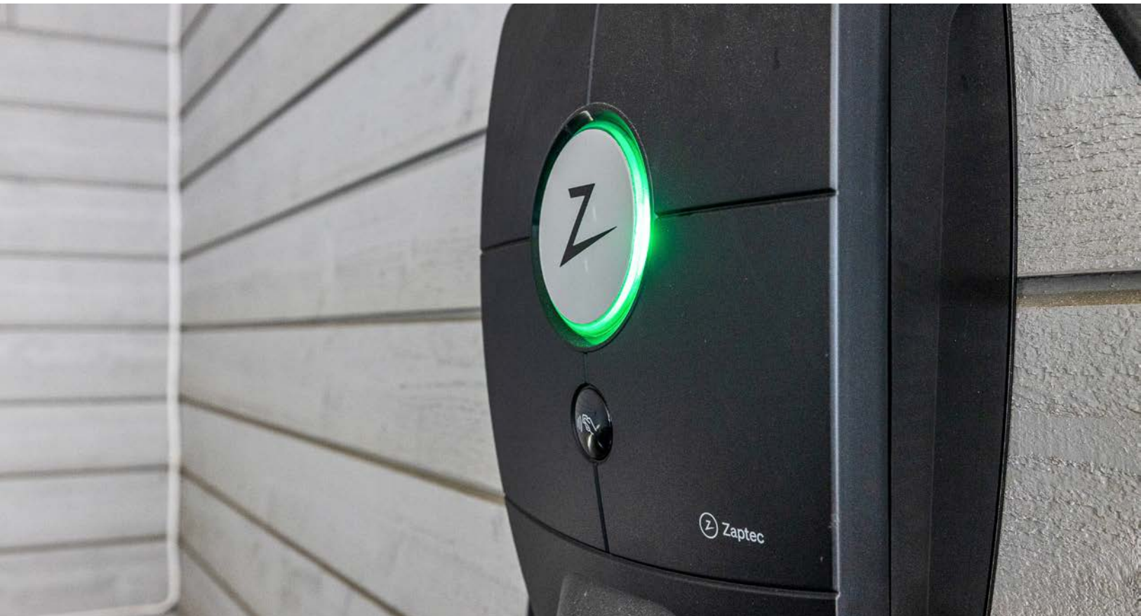
Zaptec el-bil lader i carport.
