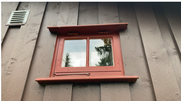
Sprekkdannelse i kitt
