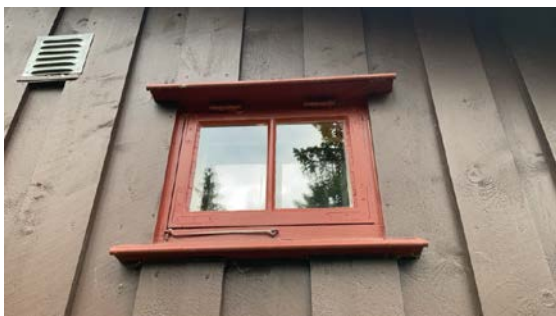
Sprekkdannelse i kitt
