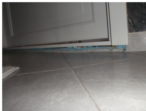
Manglende fuging under terskel
