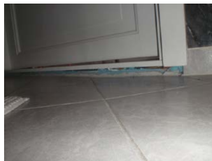
Manglende fuging under terskel
