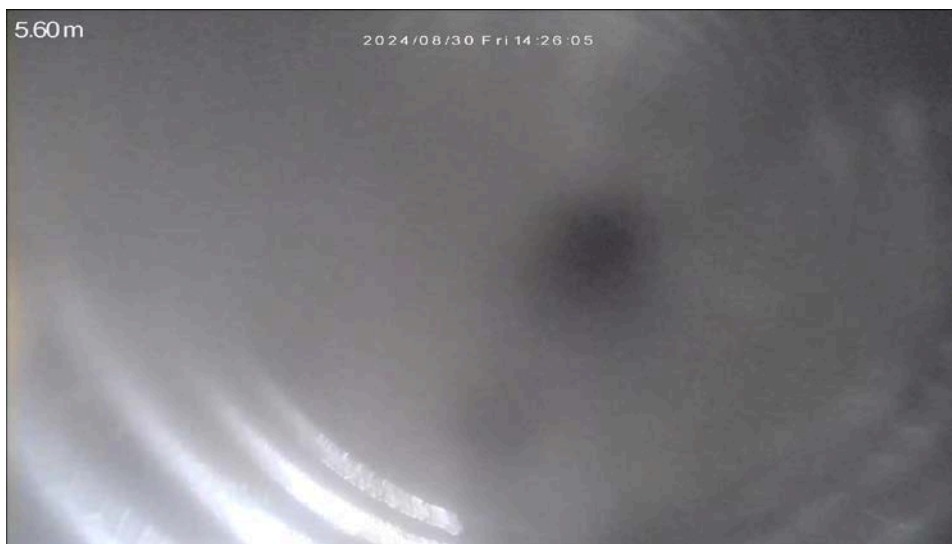
RB 5,60m Rørbrudd, Gradering 2, Type: Langsgående, KI 3
