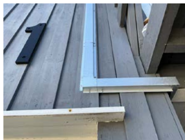
Gliper mellom trepanelet.
