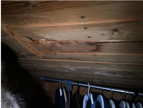
fuktskjolder himling bod 2 etg
