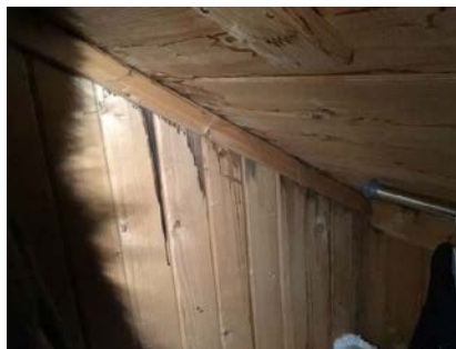
fukt skjolder himling bod 2 etg
