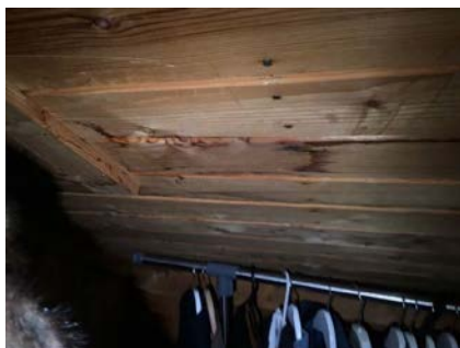
fuktskjolder himling bod 2 etg
