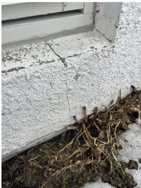
Sprekker i puss.
