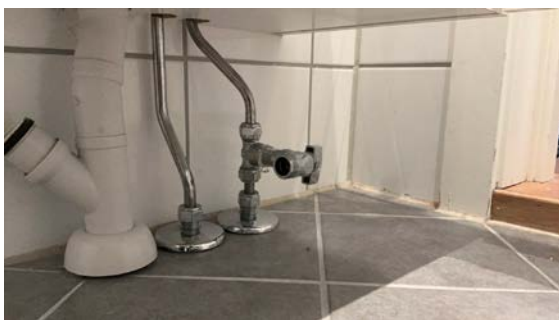
Opplegg for vaskemaskin.
