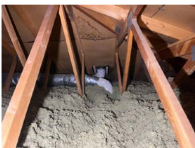
Fuktmerker i undertak plater.
