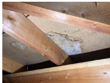
Fuktmerker i undertak plater.
