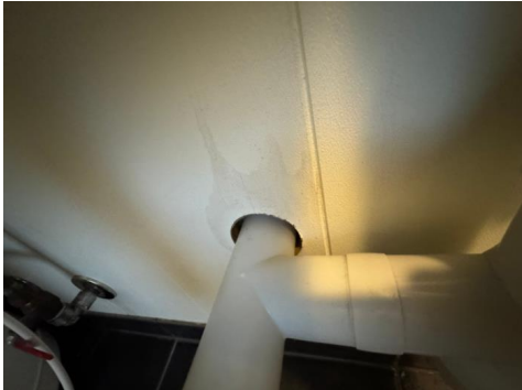
Fuktskade under servant.
