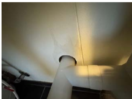
Fuktskade under servant.
