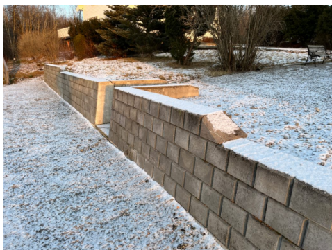
Manglende rekkverk el.
