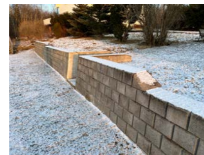
Manglende rekkverk el.
