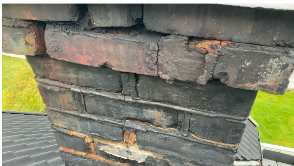
Sprekker i pipe over tak
