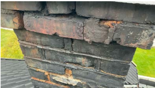
Sprekker i pipe over tak
