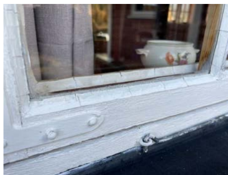
Sprekkdannelser i kitt
