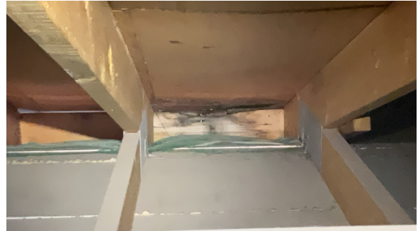
Fuktmerker i raft.
