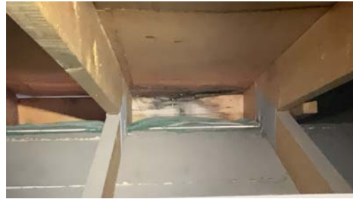
Fuktmerker i raft.
