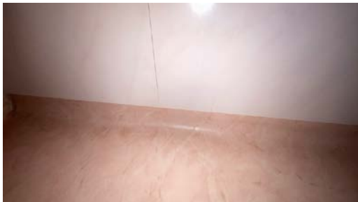
Sprekk i laminatplate under servant ned mot gulvet
