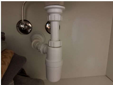
Rørpropp under servant.
