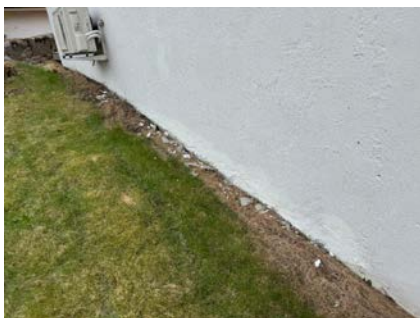
Fuktsperre delvis under terreng
