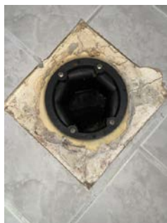
Manglende slukrist under dusjkabinett
