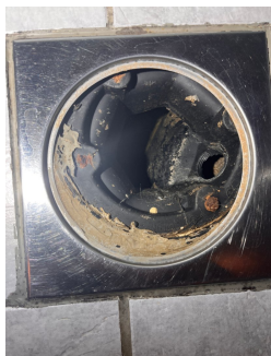
Eldre sluk, det mangler plugg sluket.
