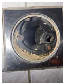
Eldre sluk, det mangler plugg sluket.
