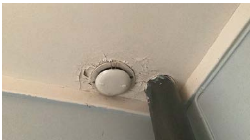
Avskaling i himling.
