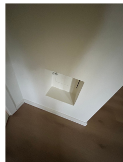
Manglende ubrennbar plate under feieluke.
