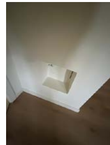
Manglende ubrennbar plate under feieluke.
