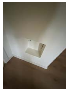
Manglende ubrennbar plate under feieluke.
