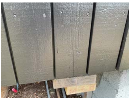
Sprekker i panel.
