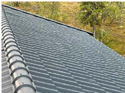
Bulker i takplater.
