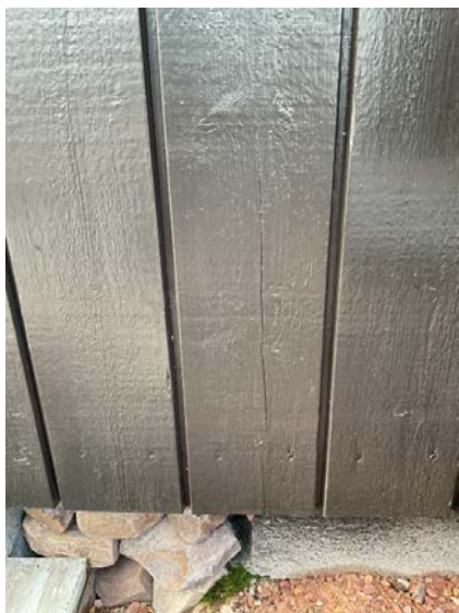
Sprekker i panel.
