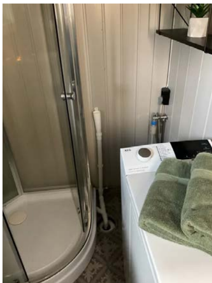
Opplegg for vaskemaskin.
