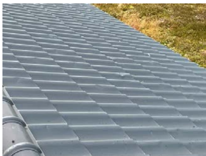
Bulker i takplater.
