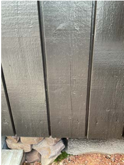
Sprekker i panel.
