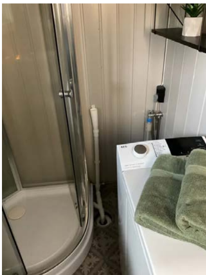
Opplegg for vaskemaskin.
