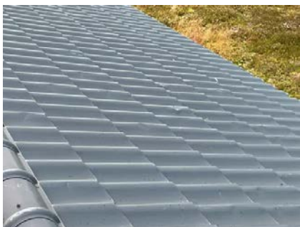
Bulker i takplater.
