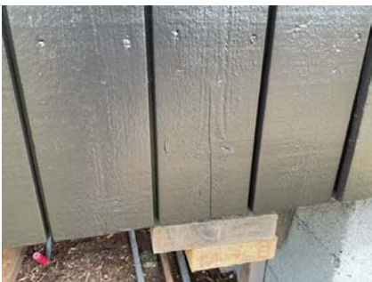
Sprekker i panel.
