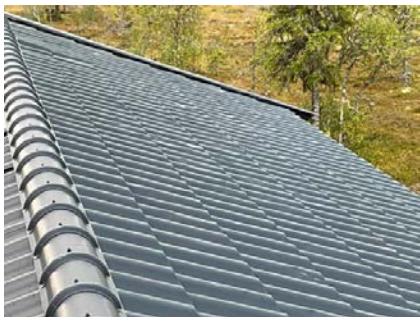
Bulker i takplater.
