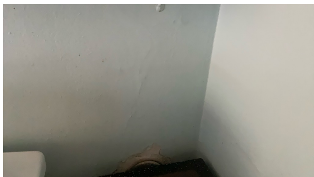
Riss/sprekker i pipe.
