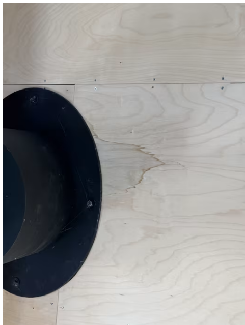
Fuktmerker rundt pipe i himling.
