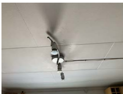
Skade i himling.
