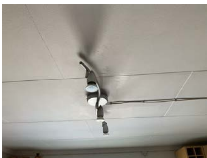
Skade i himling.
