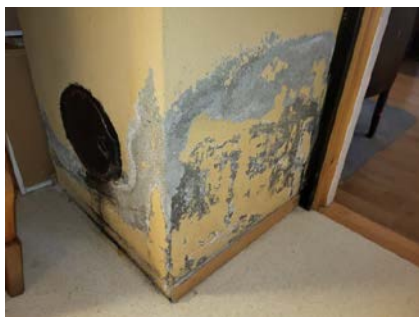
Manglende ildfast plate under sotluke
