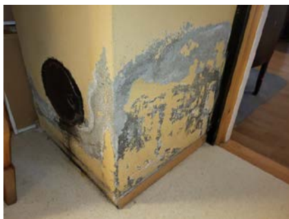
Manglende ildfast plate under sotluke
