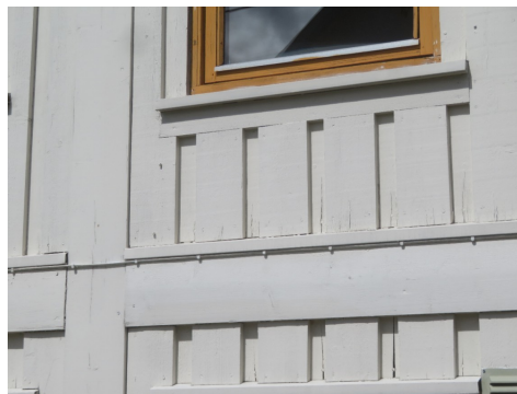
Enkelte sprekker i trepanel.
