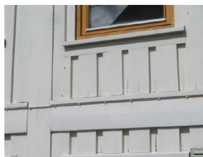
Enkelte sprekker i trepanel.
