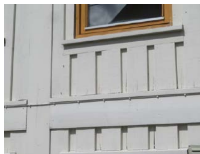
Enkelte sprekker i trepanel.
