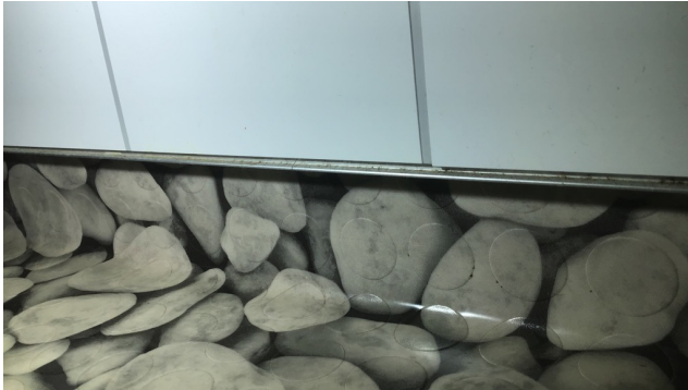
Mangelfull fuging i underkant
