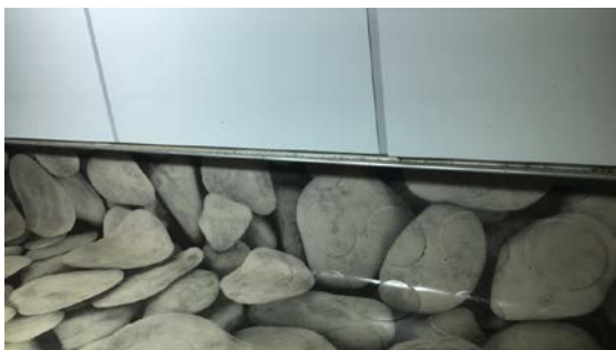
Mangelfull fuging i underkant
