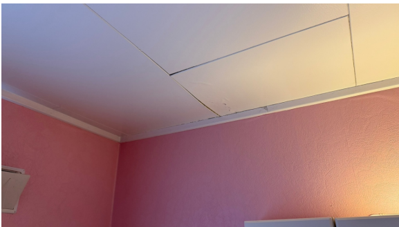
Fuktmerker i himlingen
