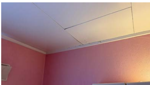
Fuktmerker i himlingen
