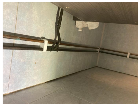
Manglende silikon i overganger.
