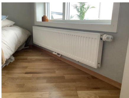
2 radiatorer for oppvarming.
